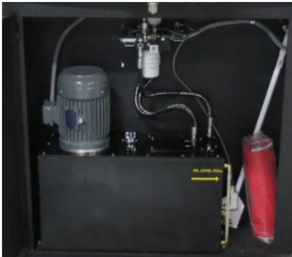
Electric Hydraulics (inside cabinet)
