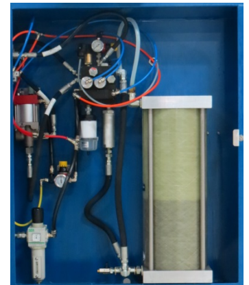
Manifold Block Hydraulics (Inside Cabinet)
